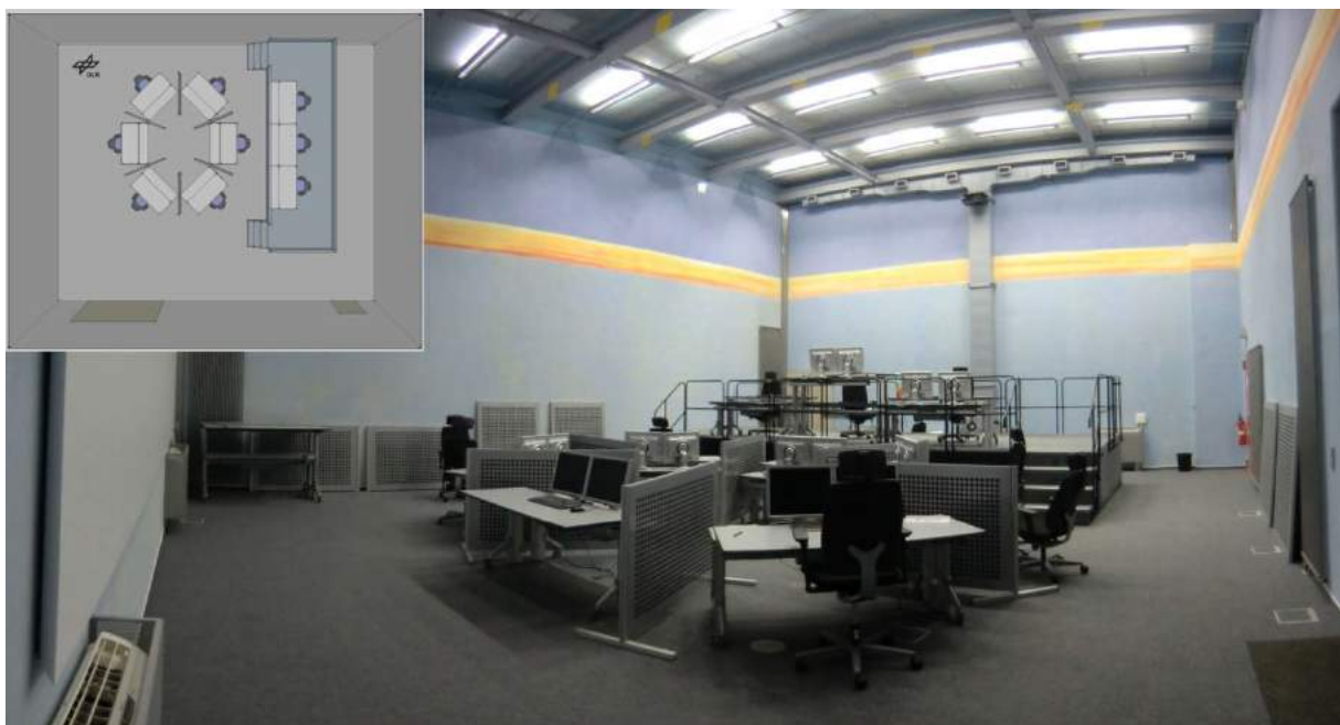
Figure 1: ACCES Control Room Layout (long shot and 2D layout, operator positions in front)
